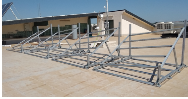
Fig. 8. Thermal solar field structure.
