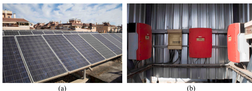
Fig. 1. PV installation: (a) BP-3165 solar modules; (b) SMC-100 inverters.
