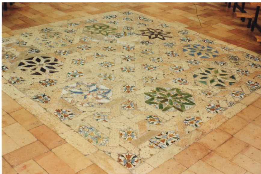
Figure 15. Brick and tile flooring. Madre de Dios Convent. Baena (Cordoba). Photo took by author.
